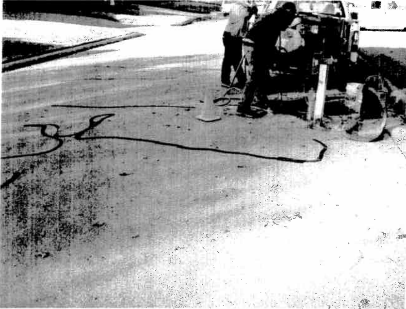
Picture #2-Sample taken from untreated area-recently crack sealed with asphalt.
